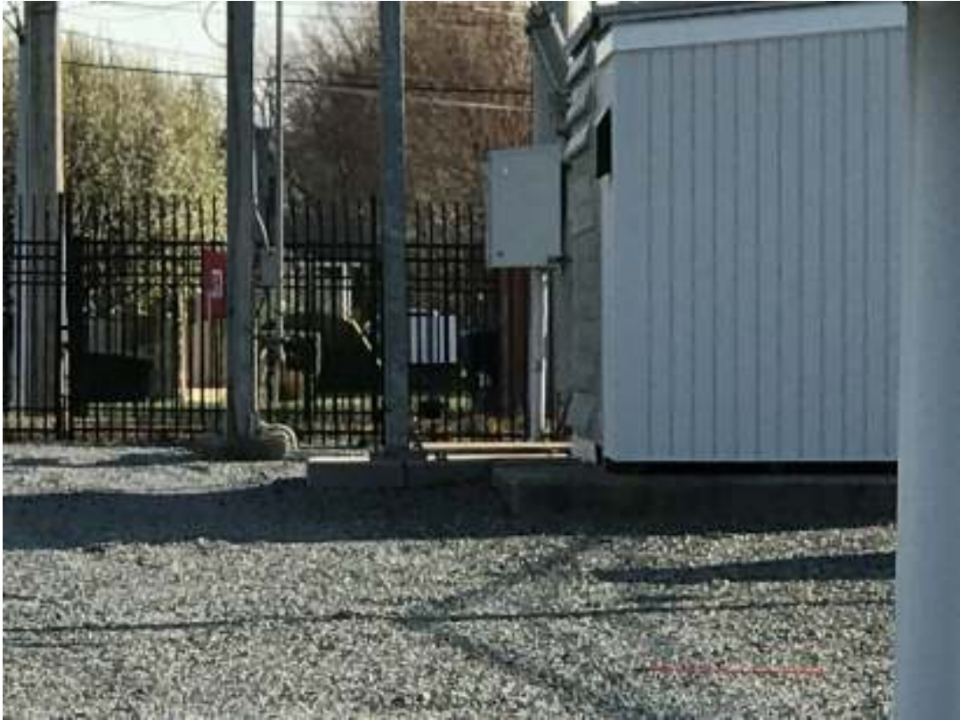
Photo 41 – Mid City Substation
