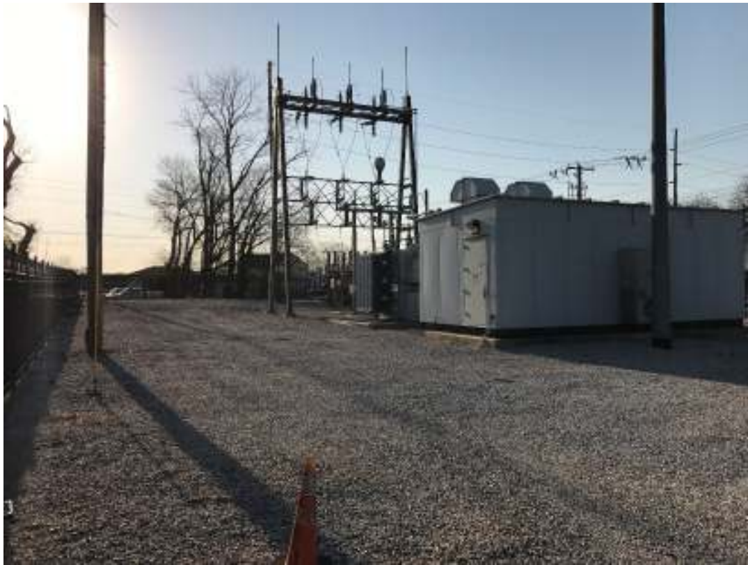
Photo 19 – Division St. Substation
