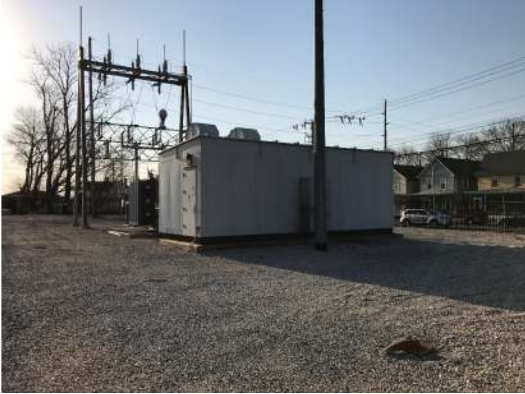
Photo 15 – Division St. Substation
