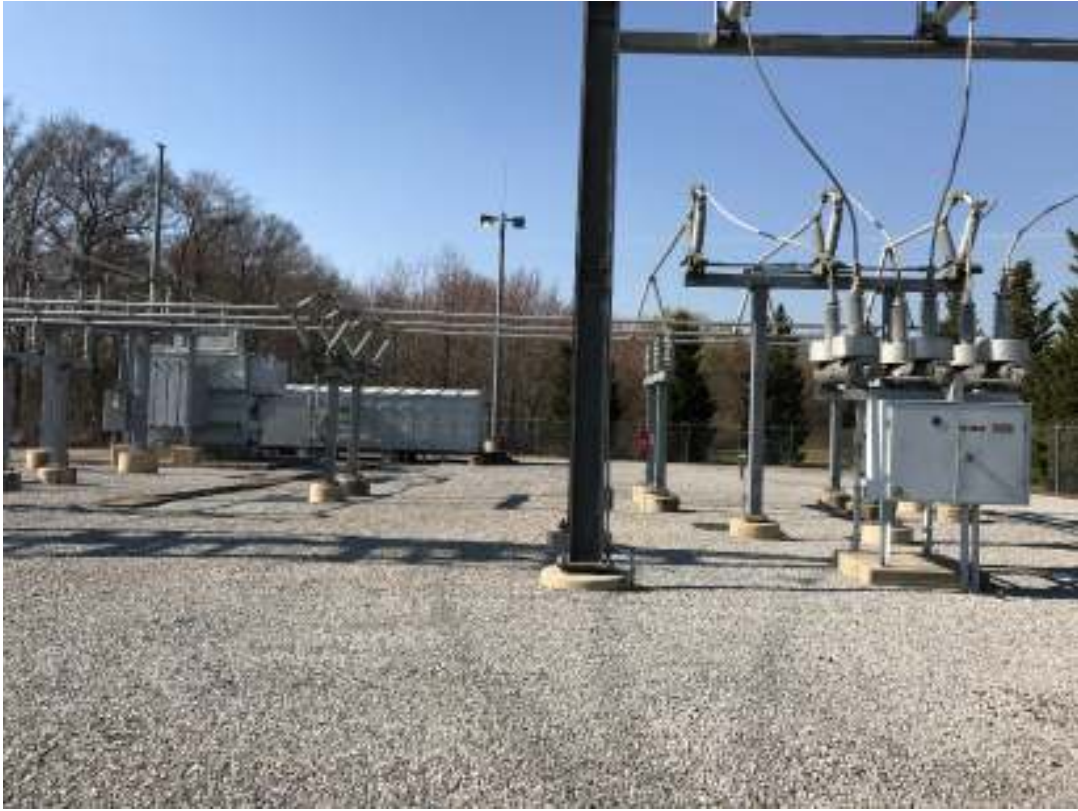
Photo 17 – Dover Downs Substation
