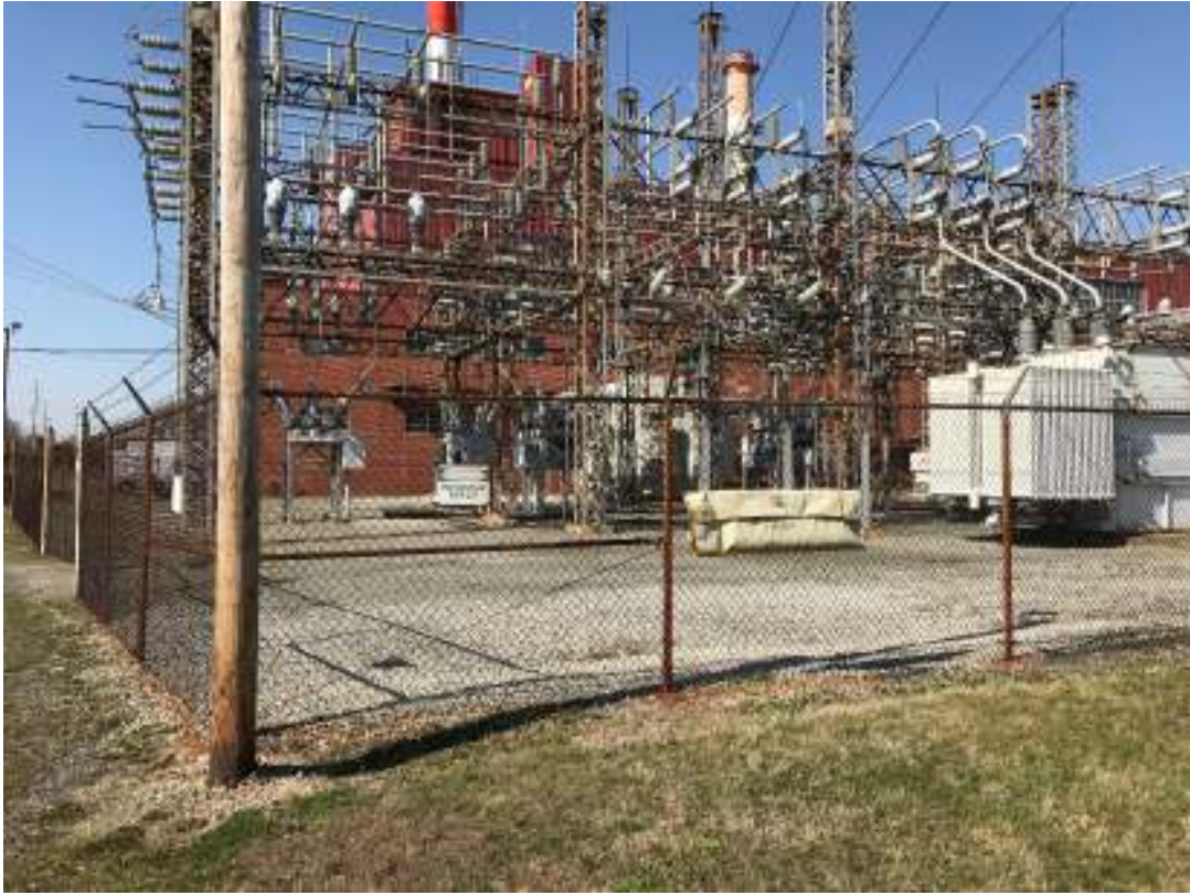
Photo 37 – McKee Run Plant Substation
