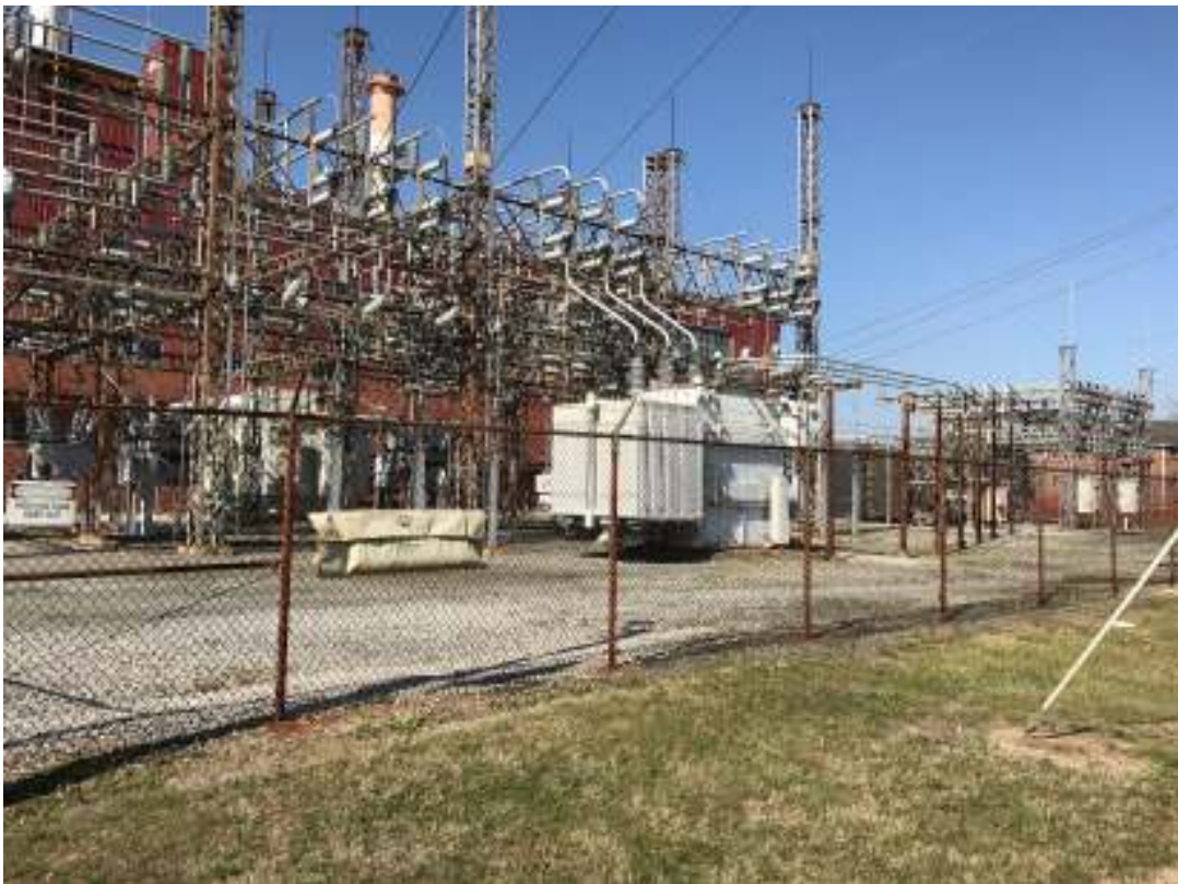
Photo 38 – McKee Run Plant Substation
