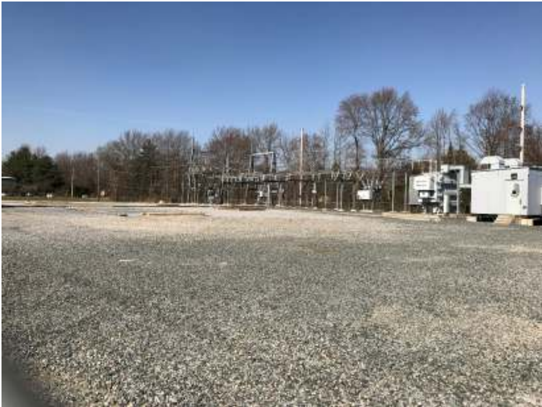
Photo 10 – College Road Substation
