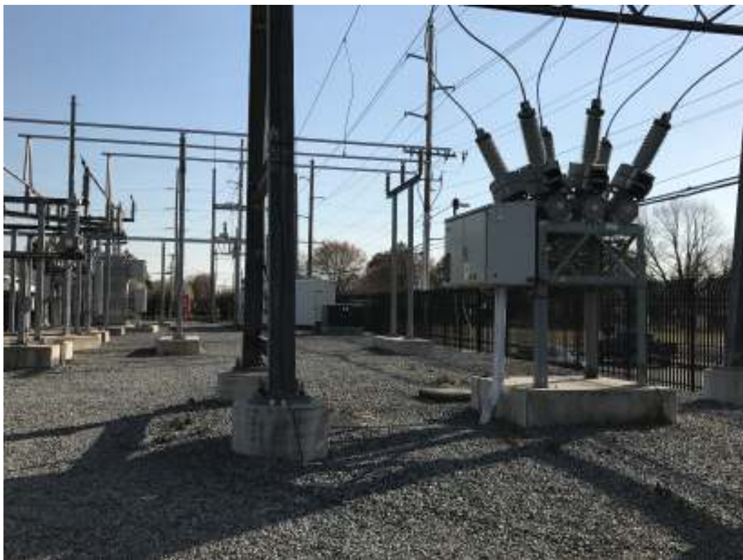
Photo 44 – Mid City Substation
