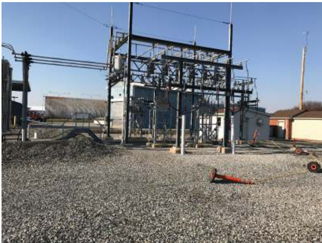
Photo 12 – Danner Farm Substation
