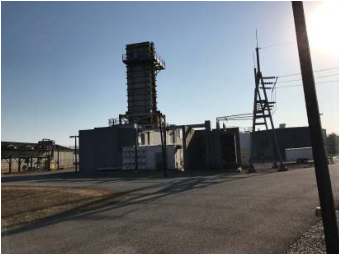
Photo 60 – VanSant Generating Station
