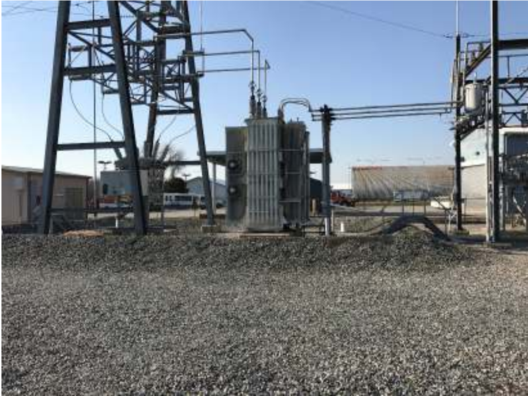
Photo 13 – Danner Farm Substation
