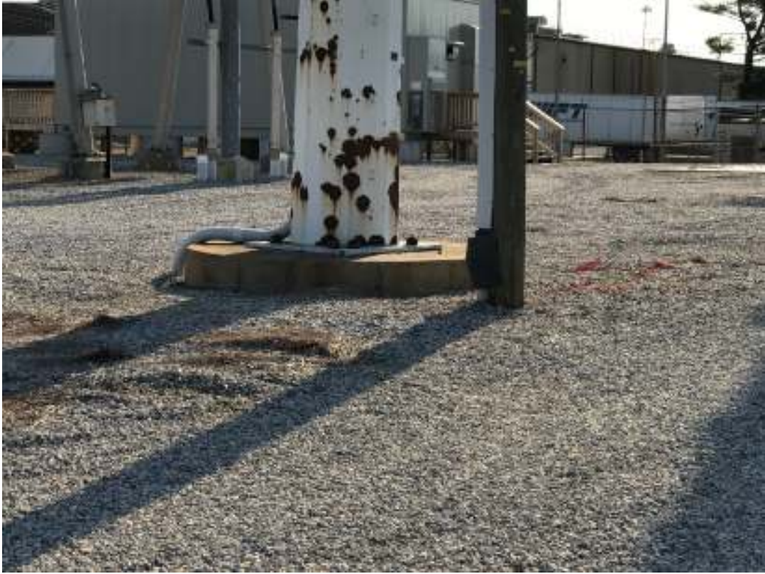
Photo 49 – North Street Substation
