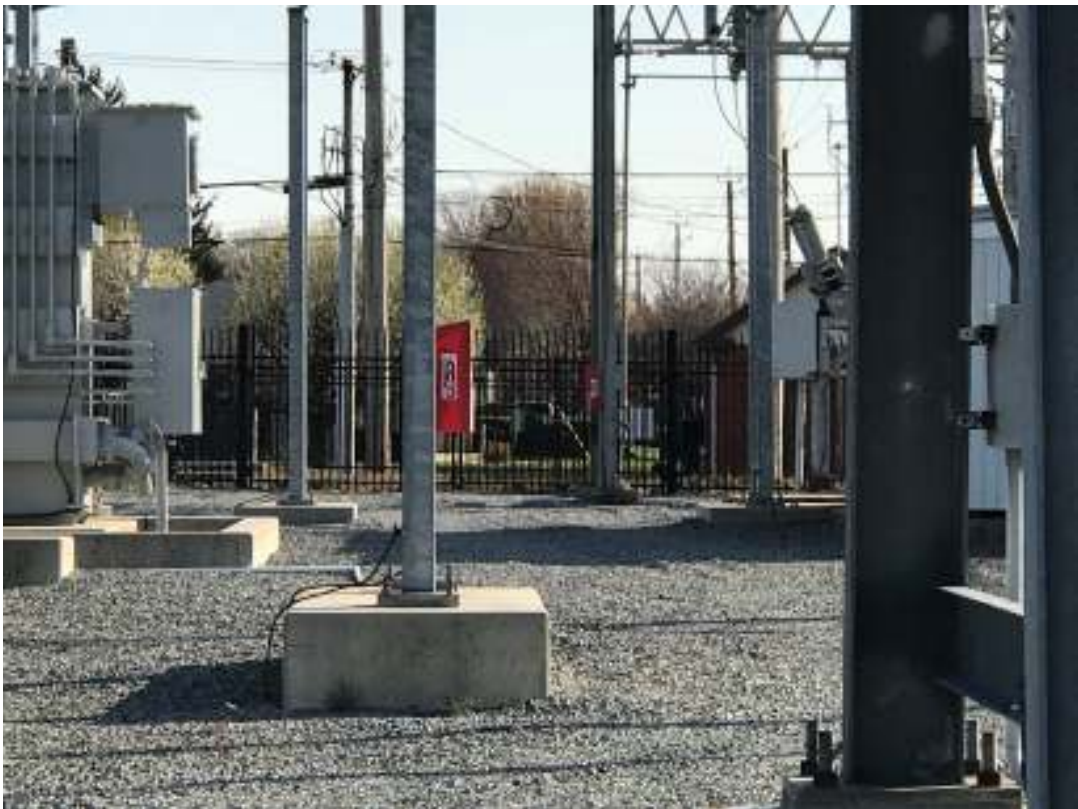
Photo 42 – Mid City Substation
