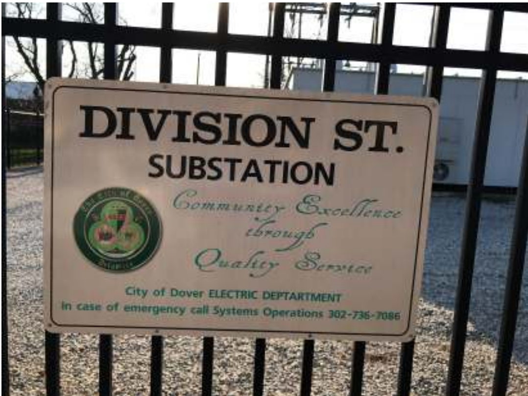
Photo 14 – Division St. Substation
