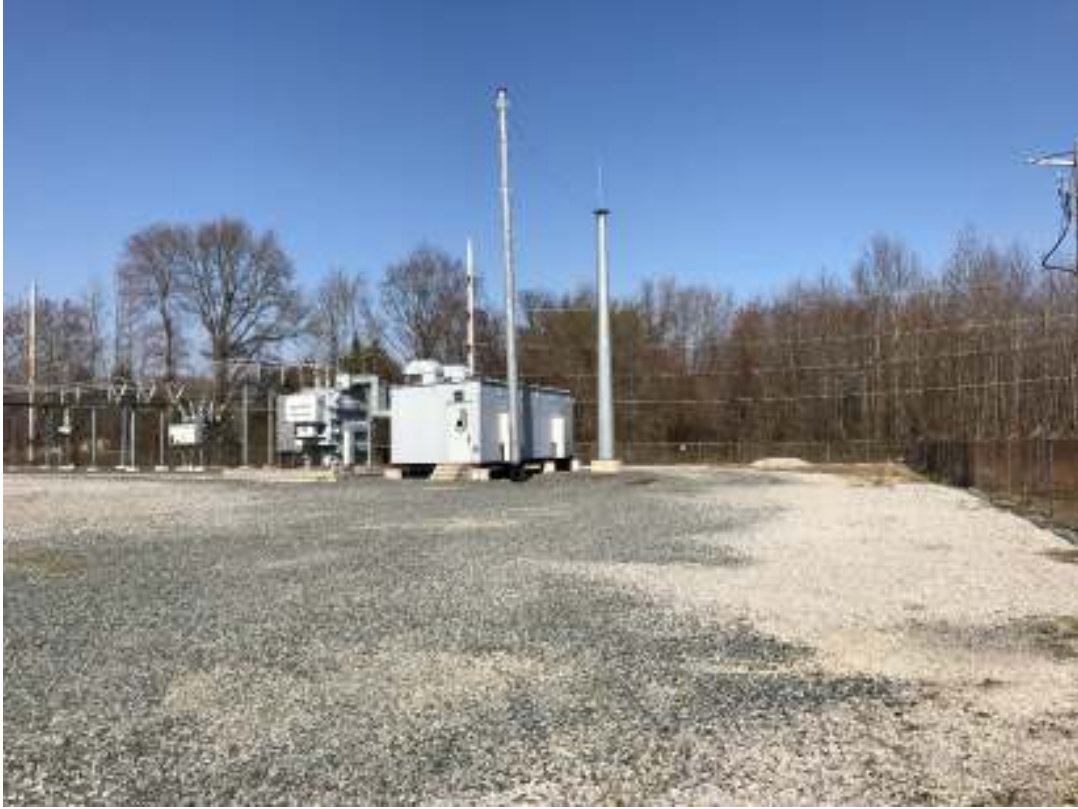
Photo 9 – College Road Substation
