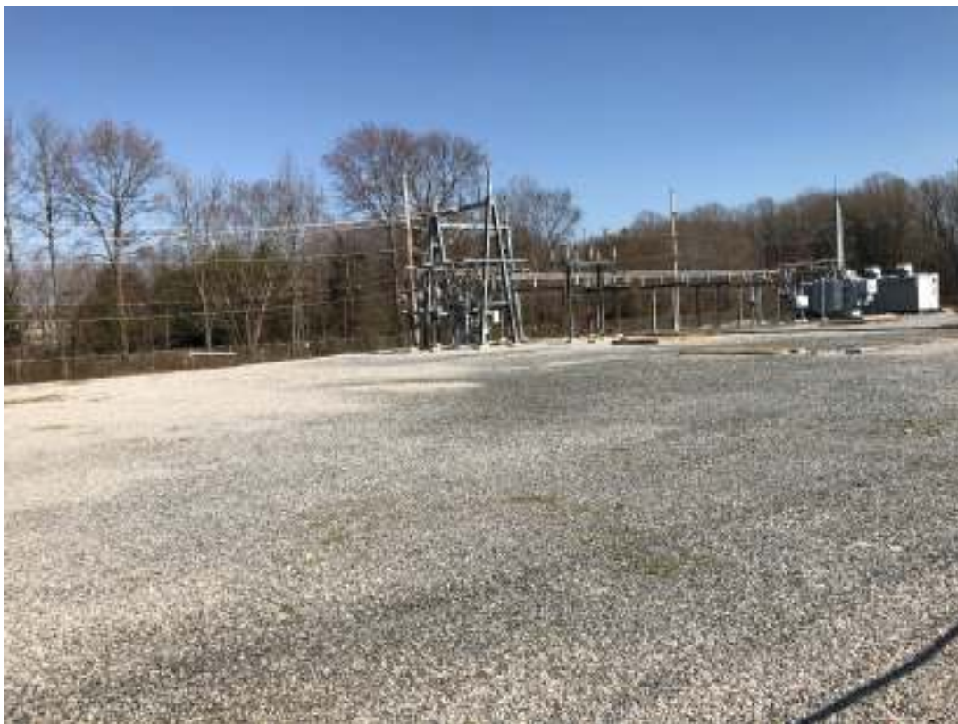
Photo 8 – College Road Substation
