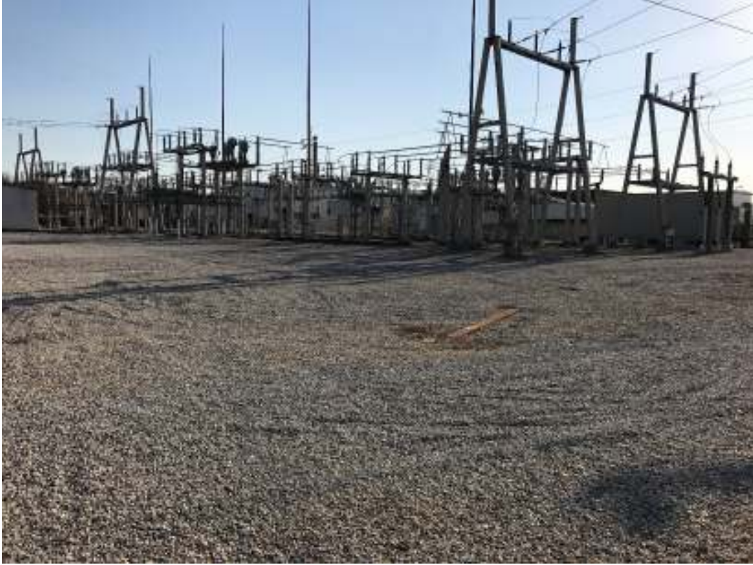
Photo 47 – North Street Substation
