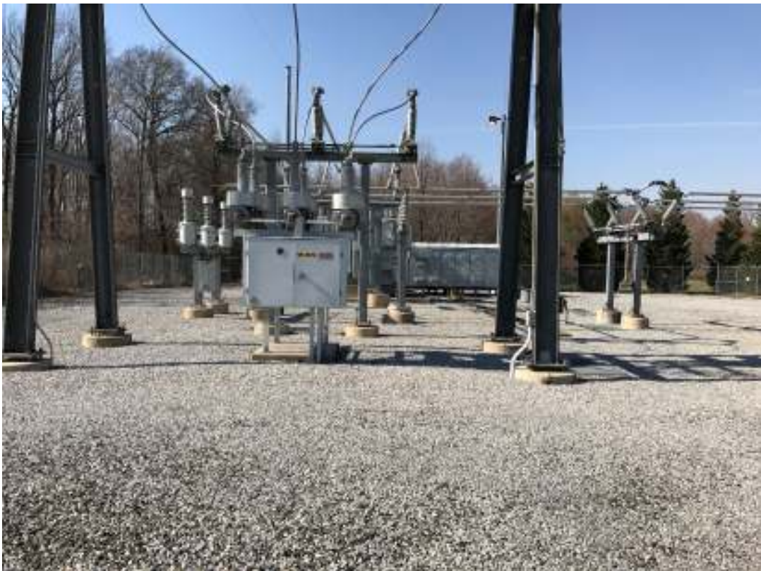
Photo 18 – Dover Downs Substation
