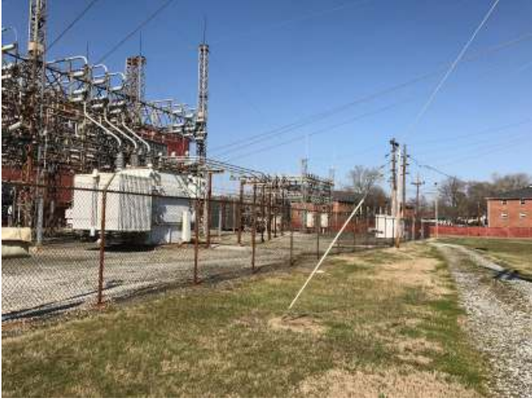
Photo 39 – McKee Run Plant Substation
