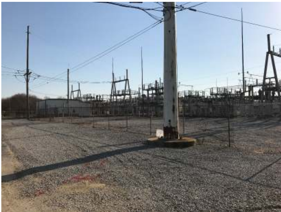
Photo 46 – North Street Substation
