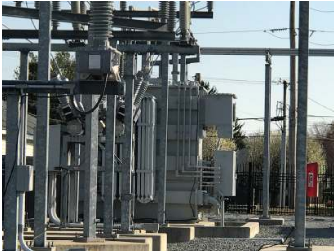
Photo 43 – Mid City Substation
