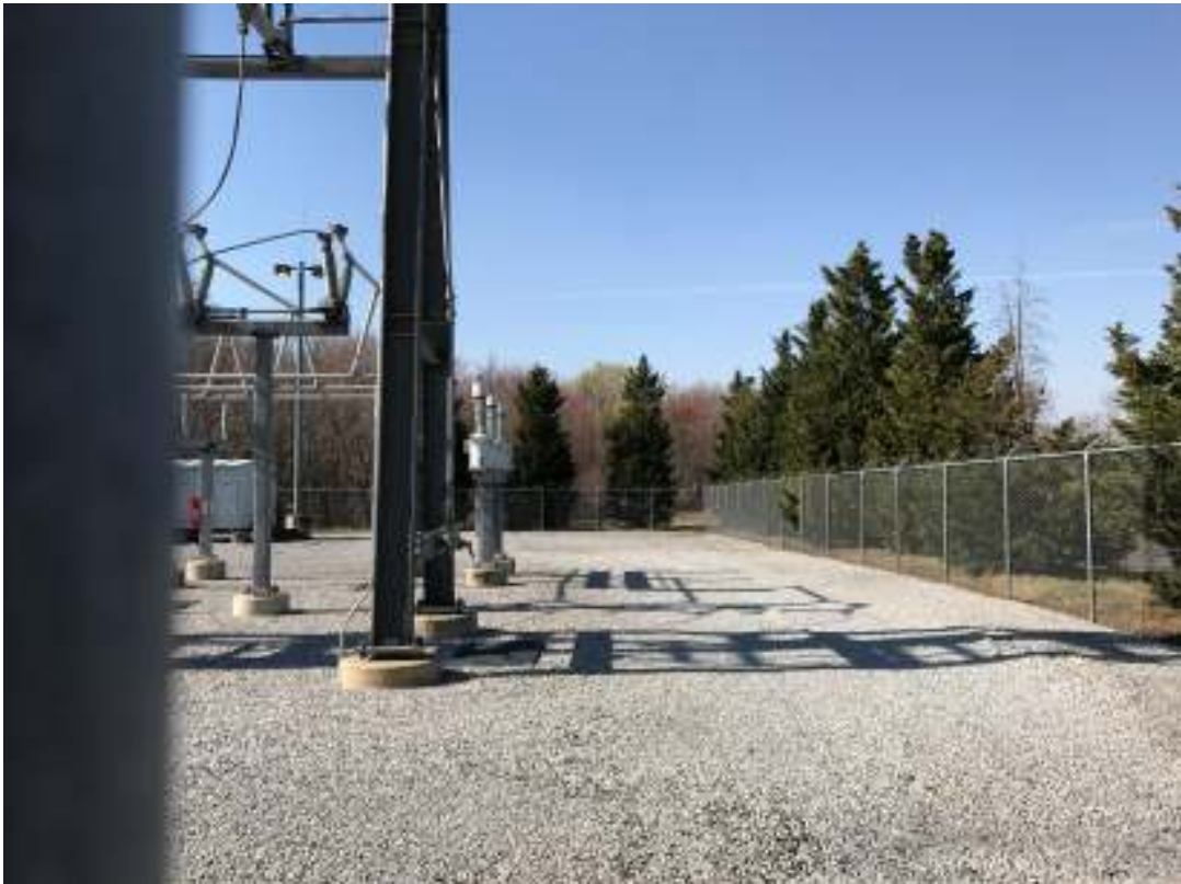
Photo 16 – Dover Downs Substation
