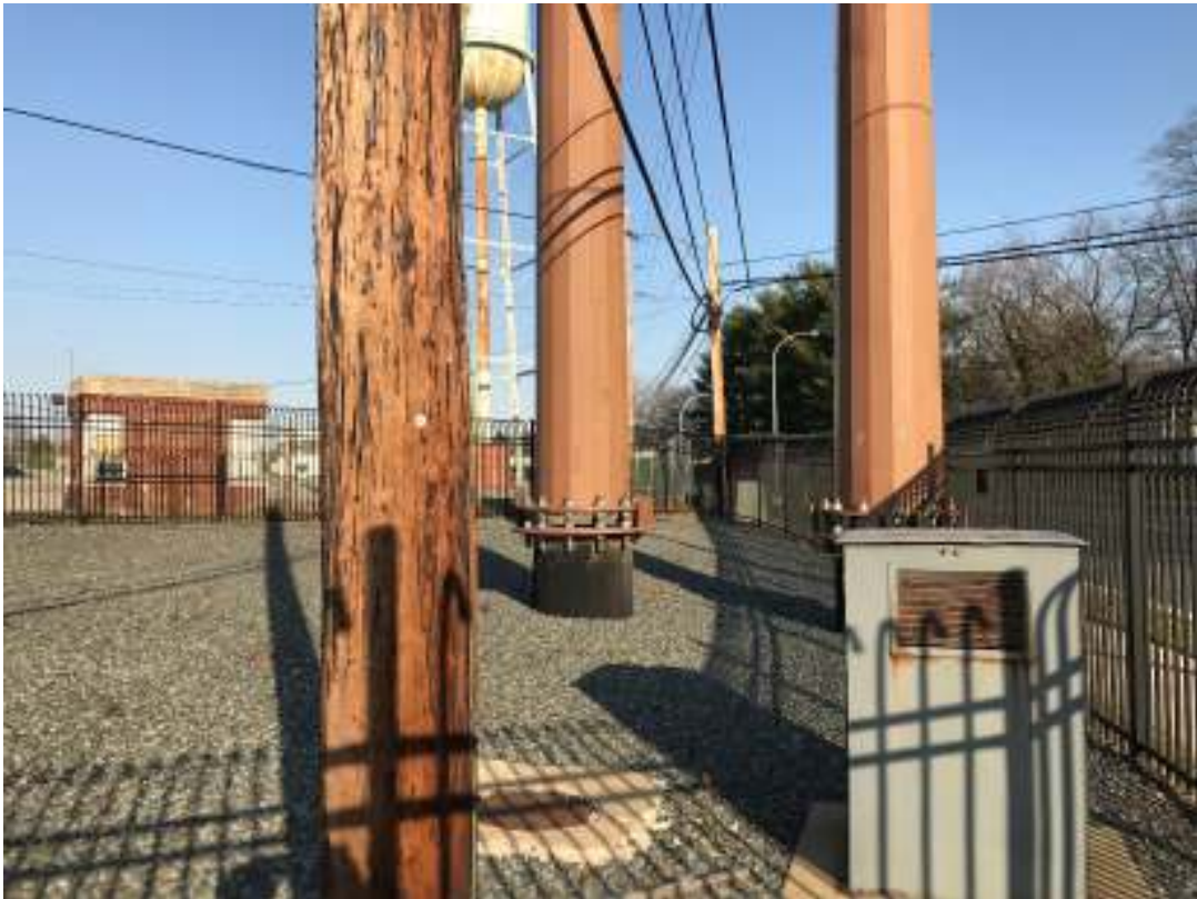
Photo 50 – St. Joan's Substation
