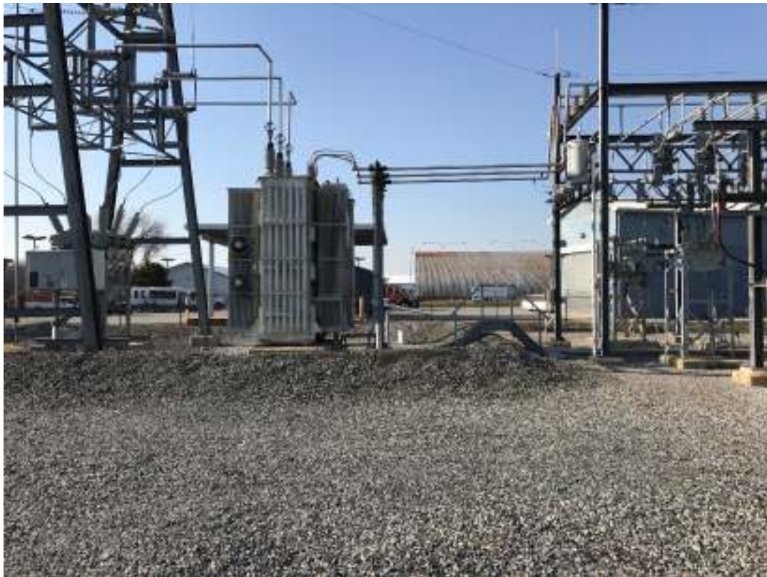
Photo 11 – Danner Farm Substation
