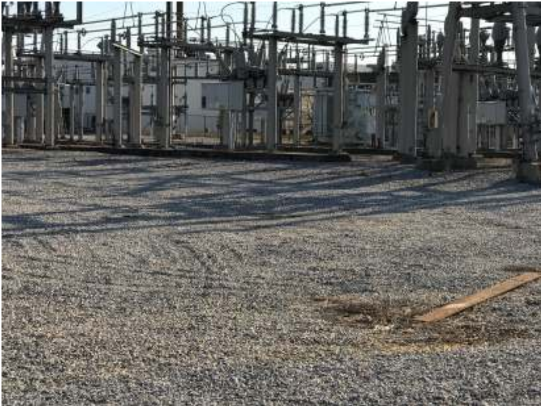
Photo 48 – North Street Substation
